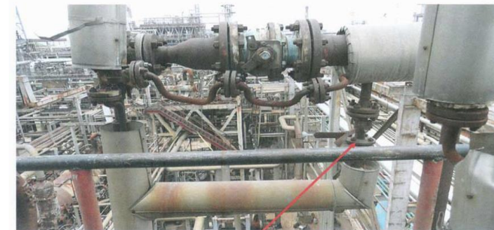
(PSV discharge line of the vessel to Flare) Bypass valve not blinded prior to opening the vessel
