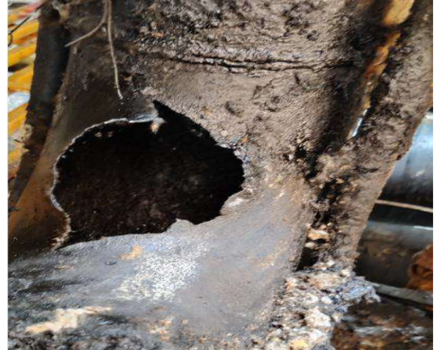
6” SR Line ruptured hole in elbow – seen after insulation removal
