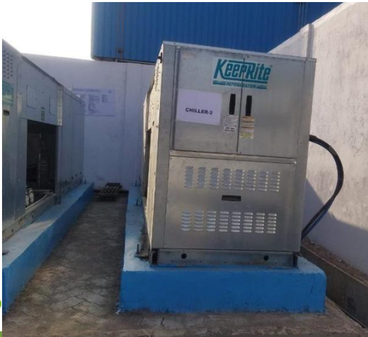
Dispenser- Chillers installed at Site
