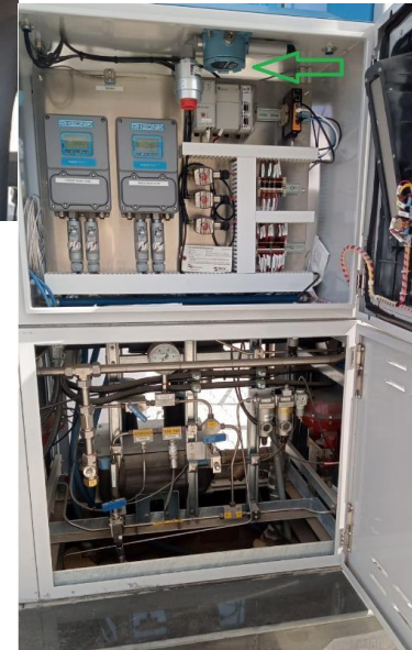
Dispenser- Gas Detector (Top Cabinet)
