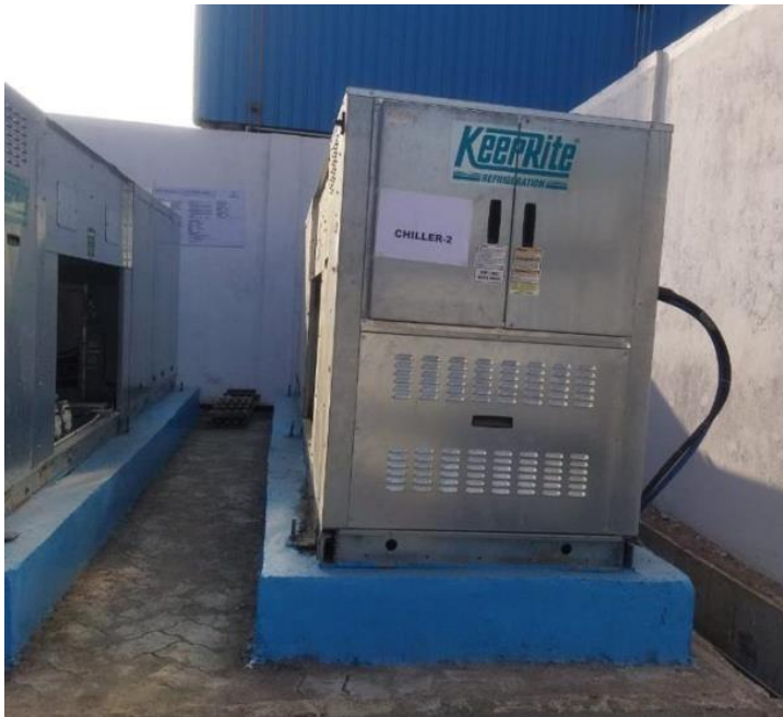
Dispenser- Chillers installed at Site
