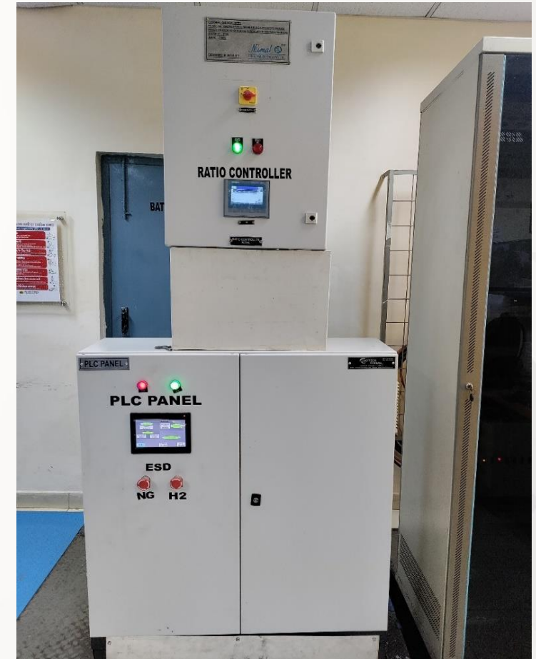
PLC Panel and Ratio Controller
