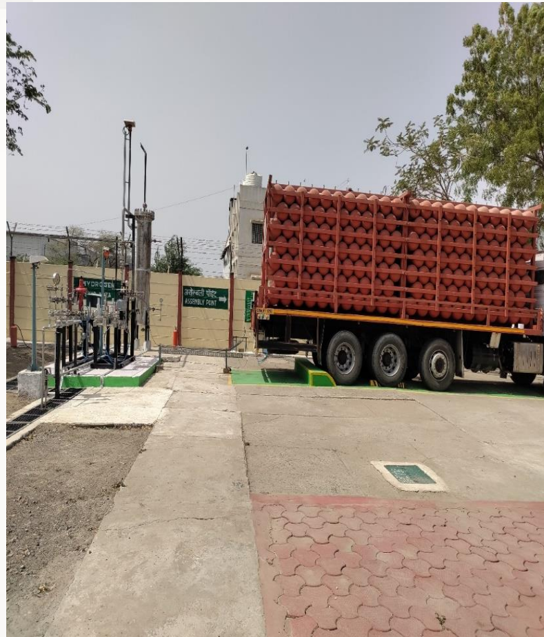
PRS skid and Cascade
