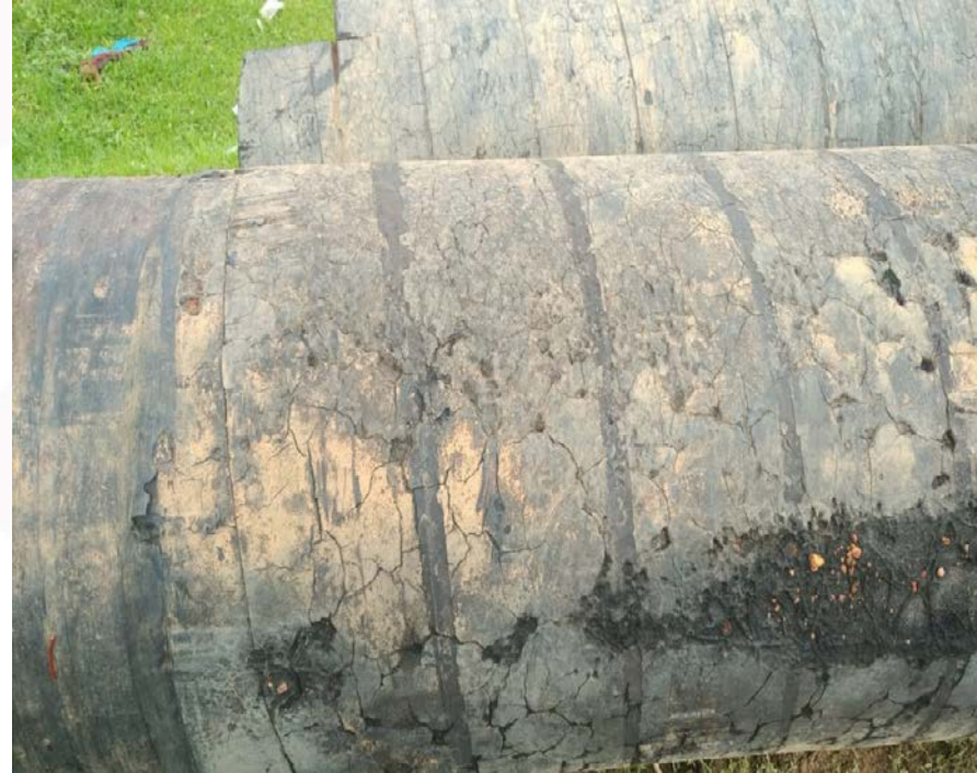
CTE AFTER 25 YEARS – CRACKING OF OUTER SURFACE
