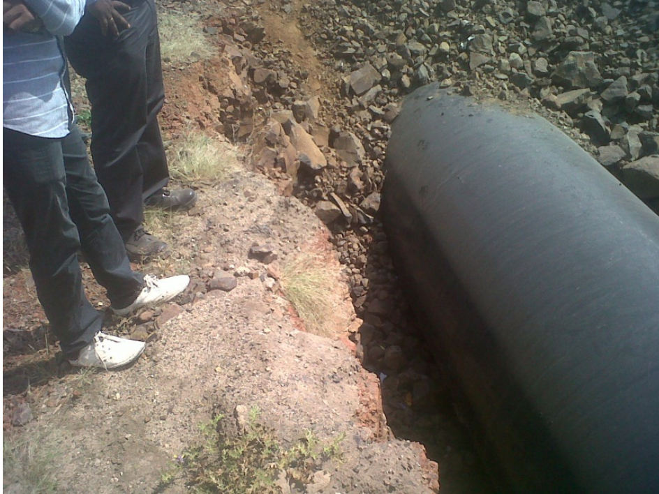
3LPE AFTER 25 YEARS – NO CRACKING OF OUTER SURFACE
