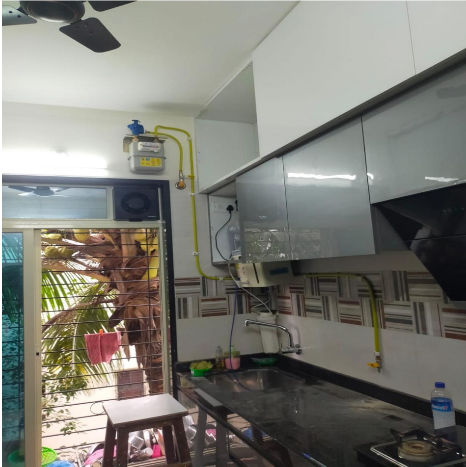
Inside kitchen Meter Installation with MLC Pipe
