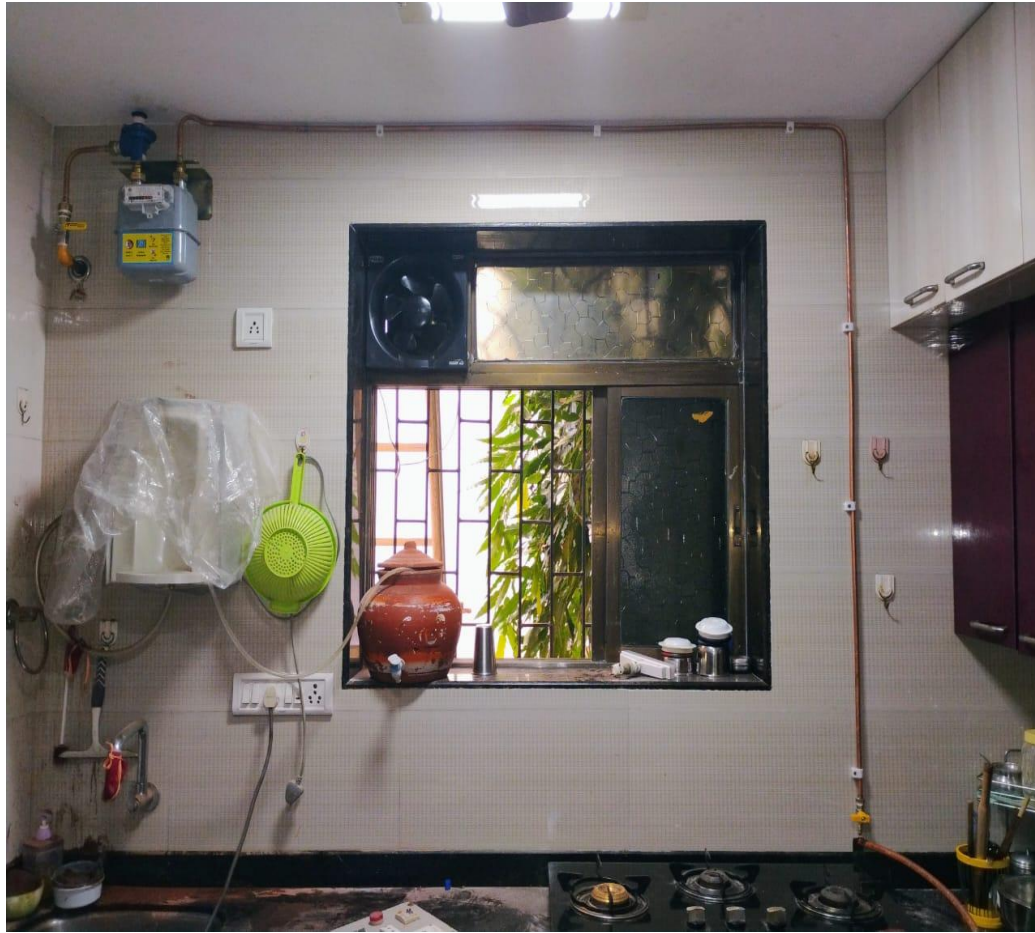
Inside kitchen Meter Installation with Copper tube
