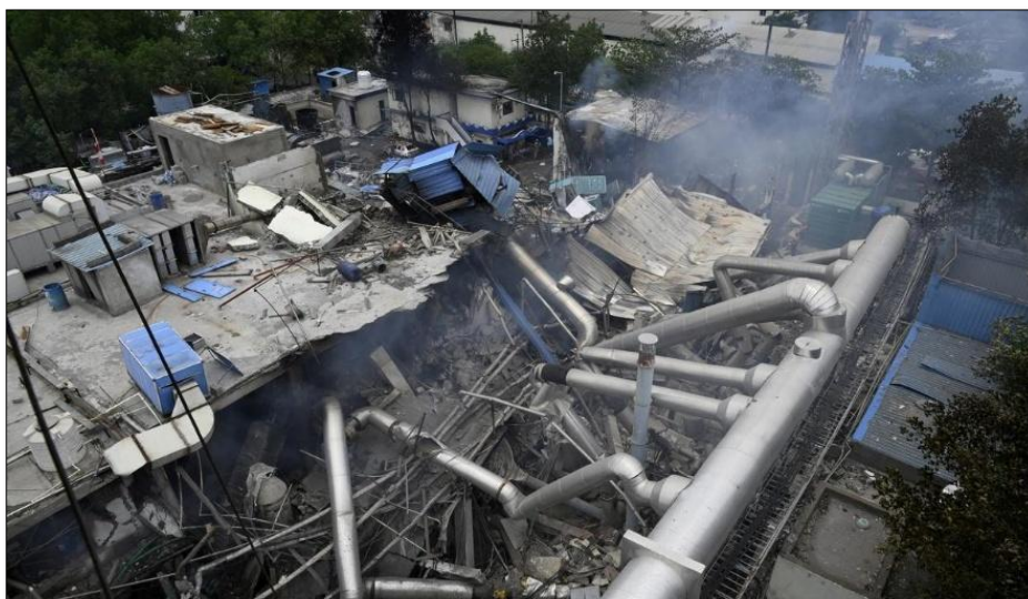
Levelled Shed after Explosion
