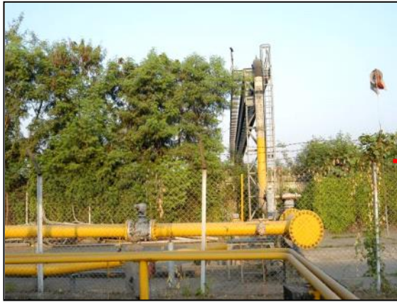
City Gate Station
