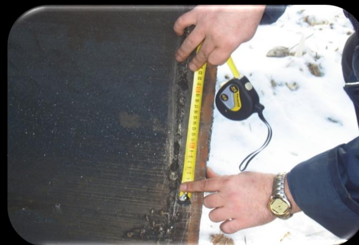
Abnormal Girth Weld
